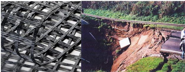
Fig. 1. Geogrid and sinkholes [1]
